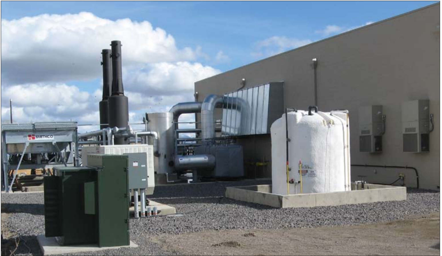
The High Sierra Cogeneration Power Plant in Susanville provides power to the Plumas-Sierra REC system and uses the waste heat from its engines to heat water for the High Desert State Prison and the California Correctional Center.
